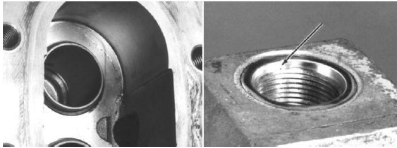
Gambar 4.13 Penampang gear body (crack)
